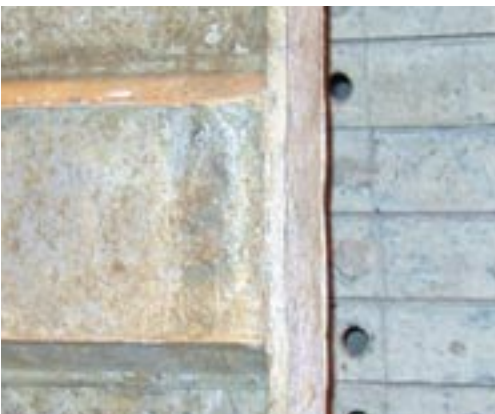
Perimeter weld breakage caused by hammer blows has caused the hat to cave in (dark depression).
