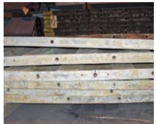
The bow on these panels will be difficult to repair.
