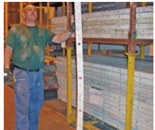
This panel was bent after a tie blowout when the crew used four ties instead of five.
