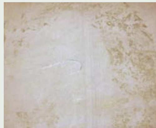
Damaged was created when a panel was dropped on to the face sheet.
