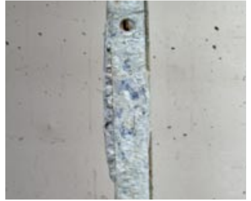
This panel gained 40 lbs when concrete seeped behind the face sheet.
