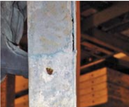
The broken welds along this siderail, caused by hammer damage, led to noticeable face sheet peel.
