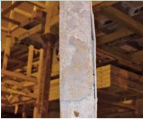
Walls poured with this form will have an ugly seam, and the concrete will seep into the panel.
