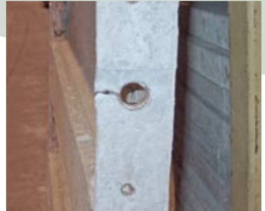
A broken siderail can lead to scrap value.
