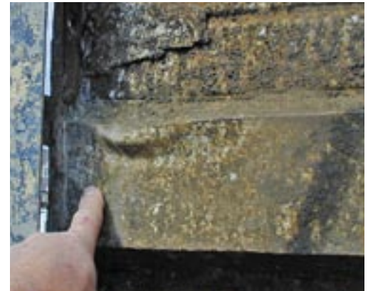
This caved-in hat section was caused by repeated hammer blows.
