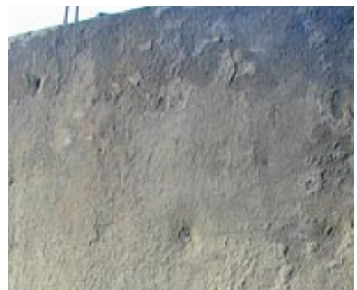
The buildup on this face sheet will lead to uneven wall finishes and added weight for the crew.
