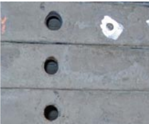
These bushing holes were altered due to incorrect tie usage (too few ties).
