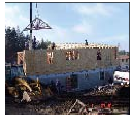
In this 2:00pm photo on Day 2, notice how the basement was already complete with windows and siding while the first floor was still being framed.
