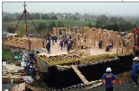
Although the middle-of-the-night pour was hard to photograph, you can see how the foundation works with the framing. And note how large the crew is to complete this project on time!
